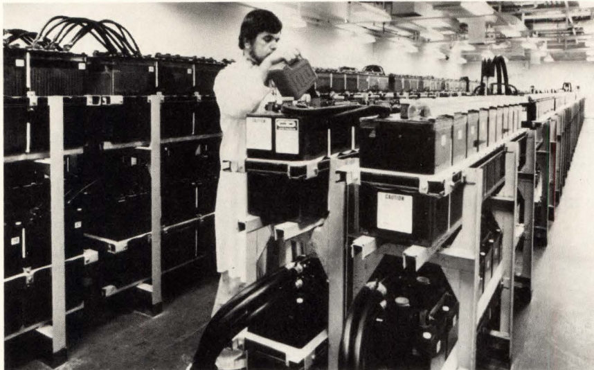
This collection of batteries backs up the UPS at Boeing Computer Services, providing a 15-minute cushion for the computer-services vendor. The batteries are by Allied Electronic Components Co.
