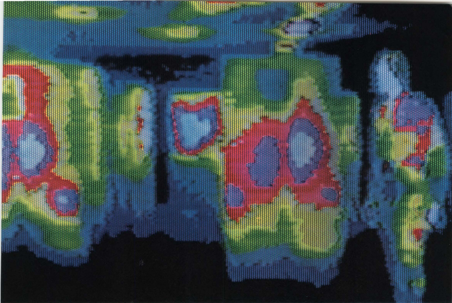
Actual infrared thermograph of a computer room.
