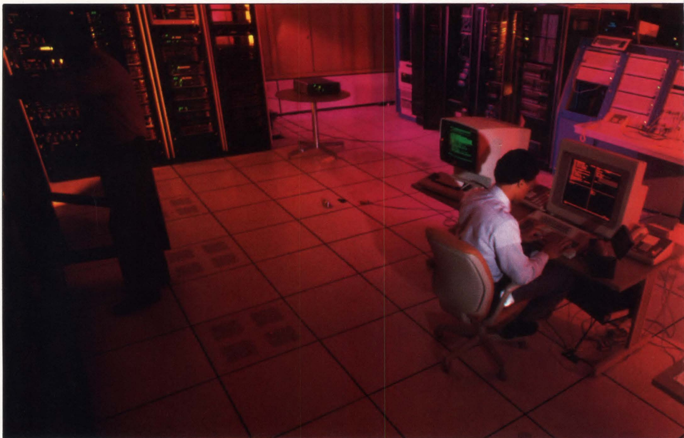
The network-control telecommunications room (above) connects First Interstate's 200 bank branches in California. Throughout the building, there are several thousand IBM 3200 series terminals that are also connected to the telecommunications network. Data are transmitted by microwave and satellite technology.
